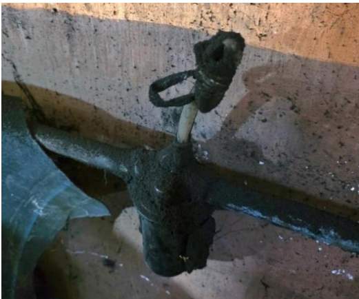
Figure 22: Airline leaks not prepared properly
