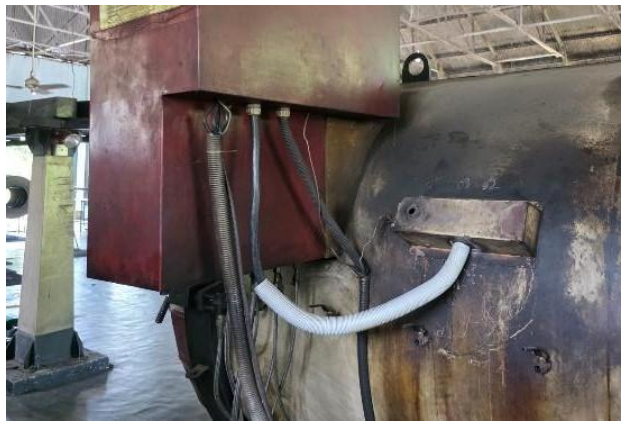
Figure 14: Improperly connected coils causing electrical sparks
