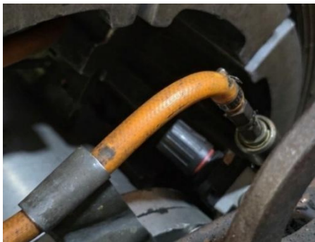
Figure 8: Pneumatic line is leaking.
