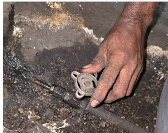
Figure 23: compressor bottom valve needs to replace
